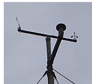
Cup anemometer on a met mast along with wind direction and solar radiation sensors.
